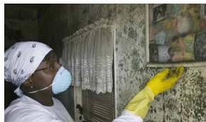
Mold on walls Credit: WA Military EMD
