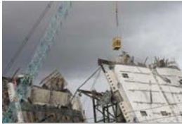
Vietnam Bridge Collapse Credit: REUTERS/Kham (Vietnam)
