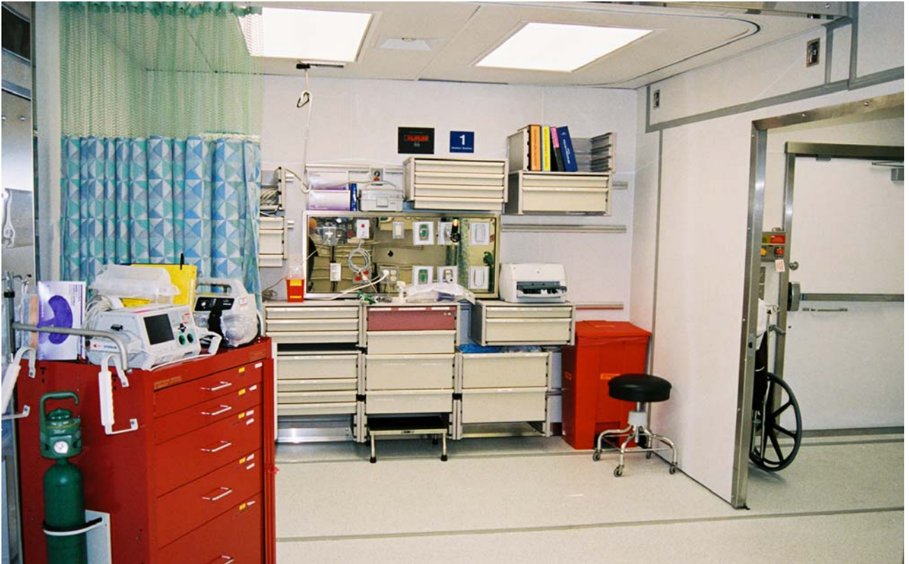
Post Op and holding area, note wide doors on right for handicap access, wheelchair lift is further right
